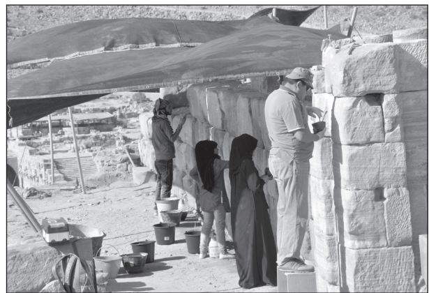
6. Conservation training in action. Mortaring of the east wall of the cella in 2016 (photo: USAID SCHEP, ACOR).
