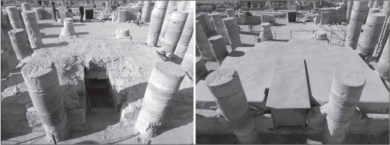
7. Before and after the application of a protective mortar capping on the cella podium in 2017 (photos: Franco Sciorilli).
